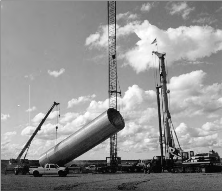
■ A 16 foot diameter structural plate shaft liner is picked up to be inserted in a bored shaft.
