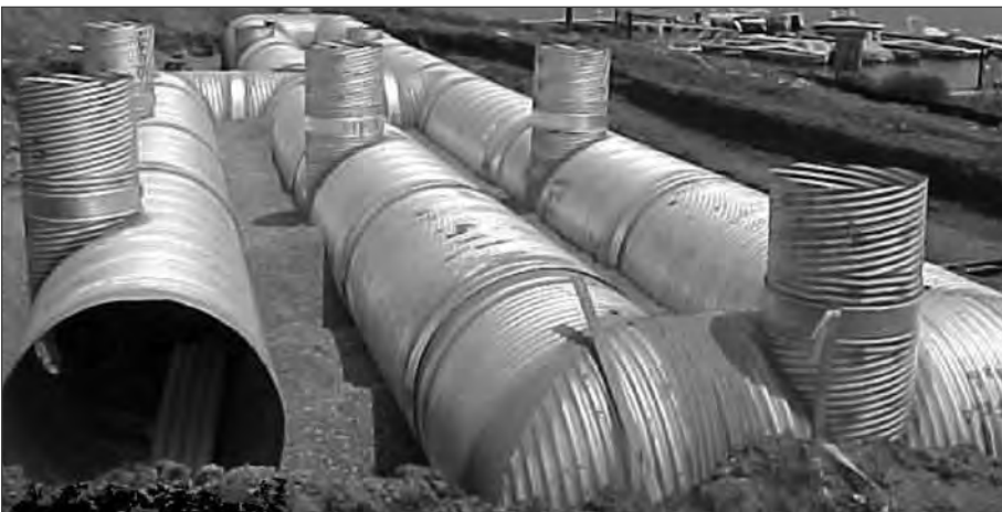
■ CSP riser manholes in underground detention system.
