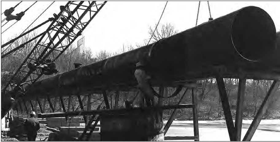
■ Corrugated steel pipe aerial sewer.
