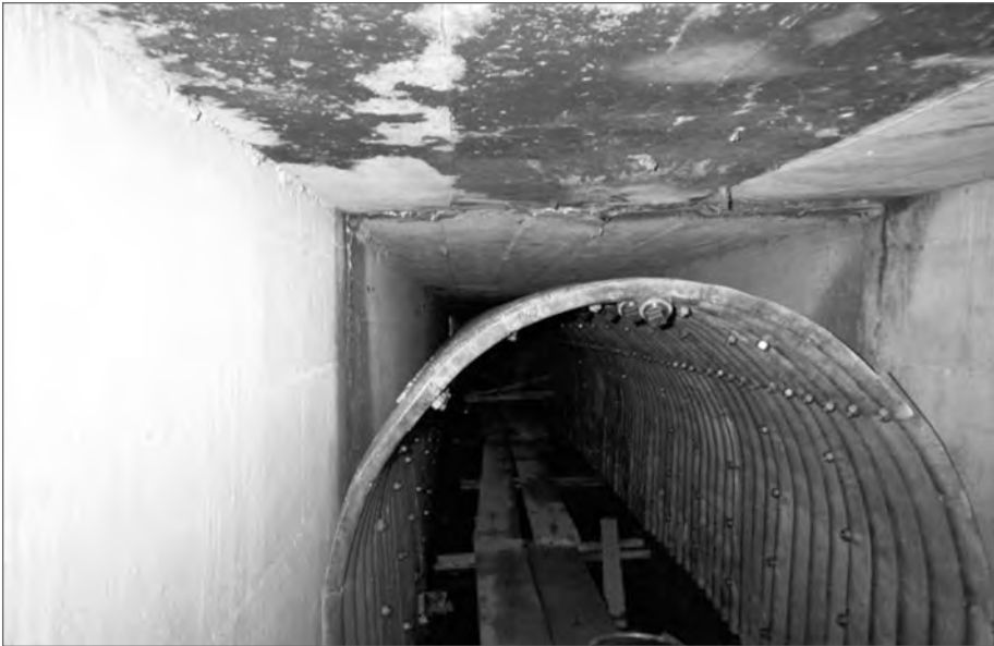
■ Figure 12.13 Structural plate arch with grout plugs used to line concrete box culvert.
