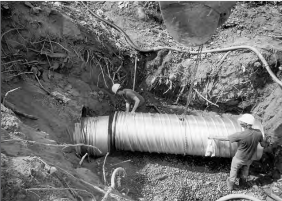
■ Figure 12.4 Pipe sections can be fabricated in lengths as required to suit slip lining installation.
