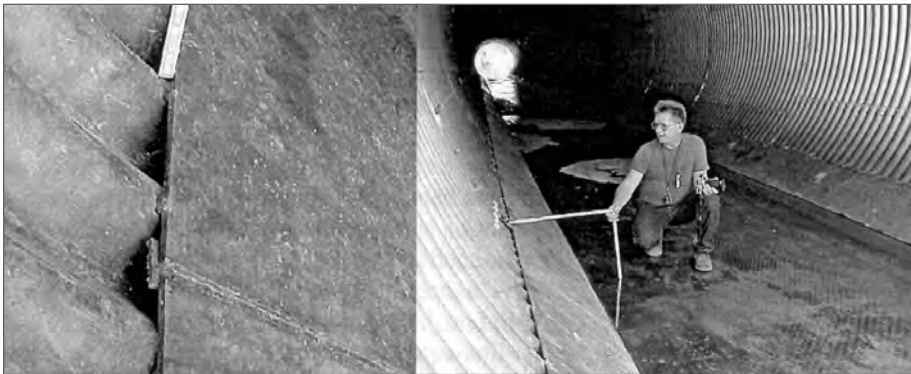
■ Figure 12.16 Steel armor-plated invert.
