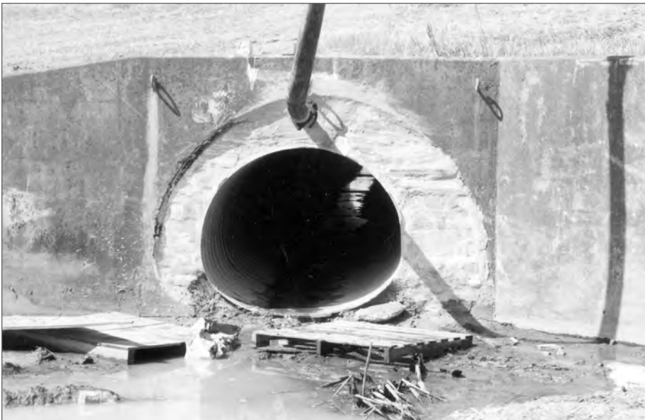
■ Figure 12.14 Grout can be pumped into annular space through an opening in the end bulkheads.
