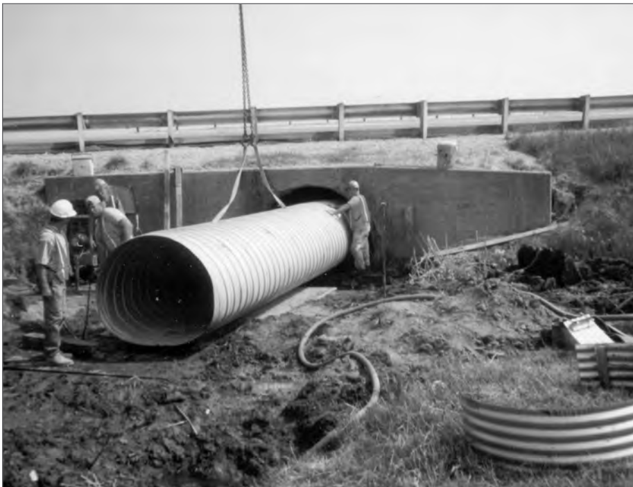
■ Figure 12.3 Typical slip lining installation with a pipe arch shape to suit existing cross-section.
