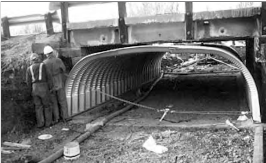
■ Figure 12.7 Deep corrugated box culvert lining a falling bridge. Note the dozer pulling the corrugated box culvert into position.
