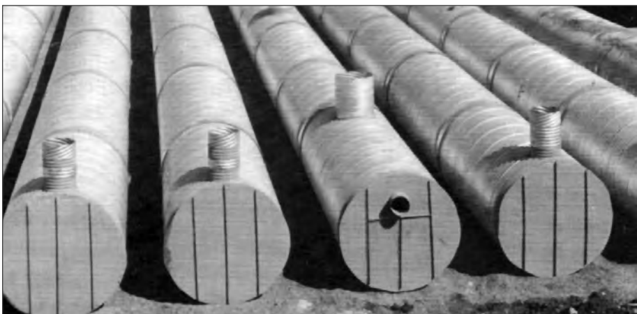
■ Figure 11.2 Seven lines of 96 inch CSP being installed to form an underground stormwater detention facility.
