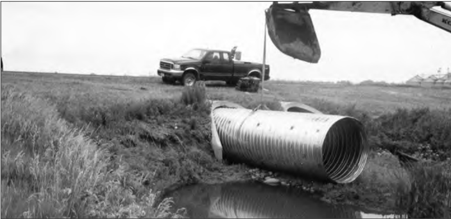
■ Figure 11.5 There are many economical pipe rehabilitation techniques being used. One method employs the use of CSP to slip line distressed reinforced concrete pipe.
