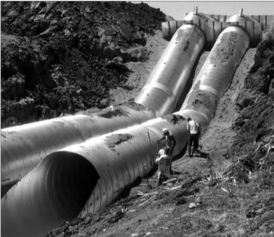
■ Installation of a corrugated steel pipe spillway. Note the anti-seep collars on the pipe.
