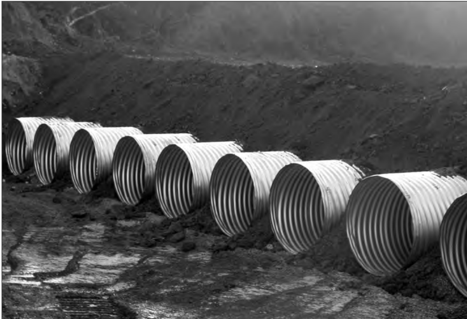
■ Multiple lines of CSP provide an effective low profile culvert crossing.
