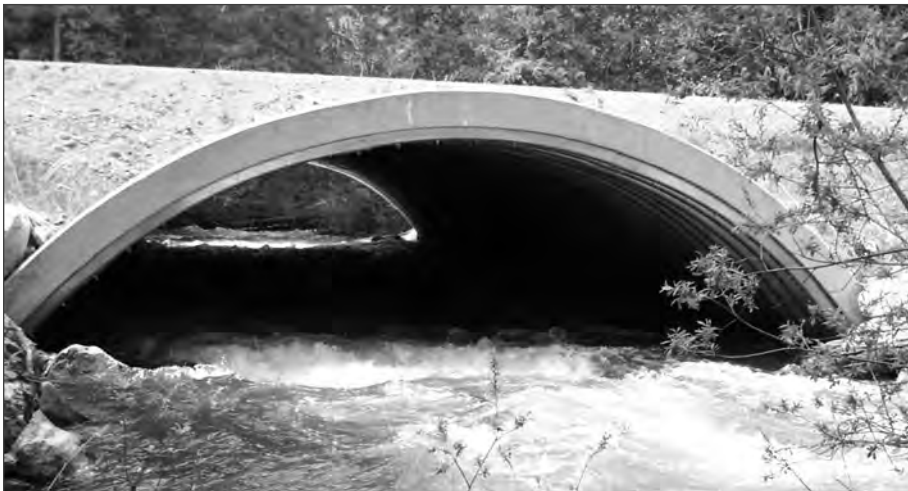
■ CSP arch preserving natural stream bed for fish passage.
