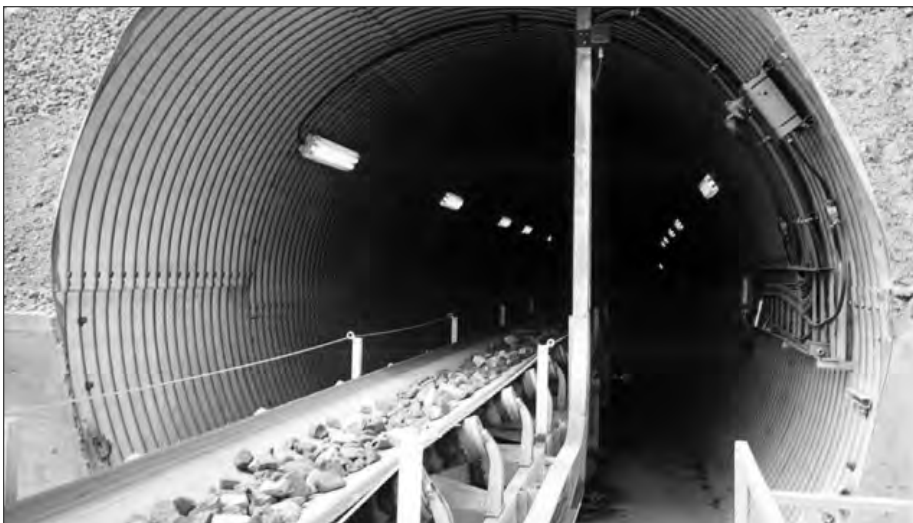
■ Conveyor crossing and walkway access for aggregate handling facility.
