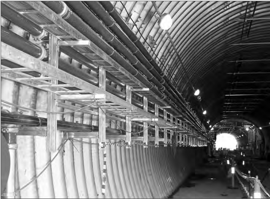
■ Corrugated steel utility conduit.
