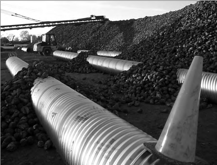
■ CSP ventilation system for sugar beet storage facility.
