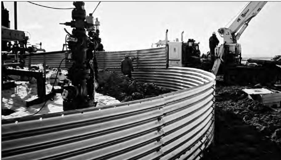
■ Corrugated steel rings used for spill containment.
