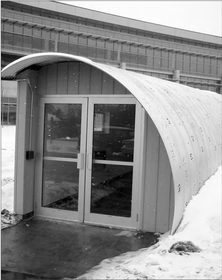
■ A section of CSP used for an entry way.
