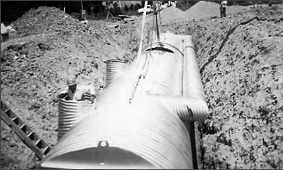
■ Effective water quality is attained by using an underground CSP sand filter.
