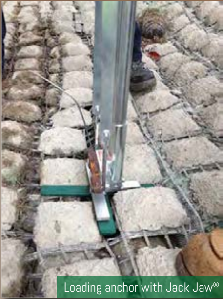
Gas powered driver installation.
