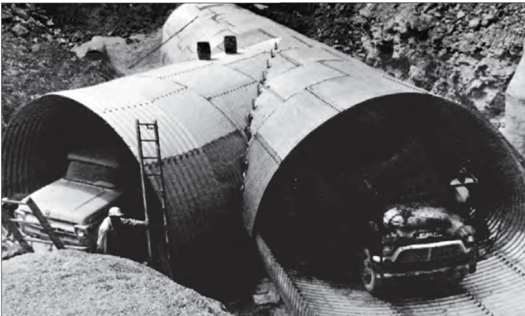
■ King-size wye or lateral for large storm sewer was shop-assembled, then dismantled and shipped to the job site for final erection.
