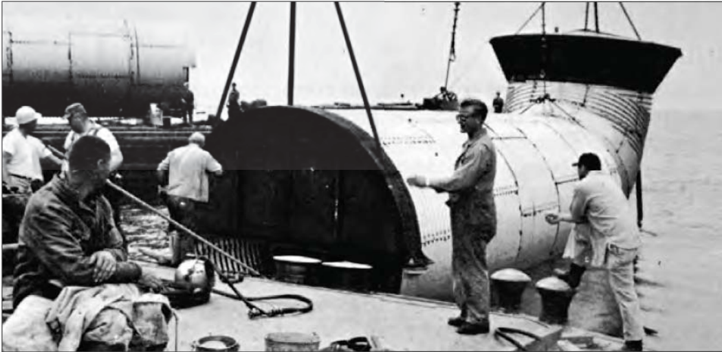
■ Special galvanized steel fitting for lake water intake of power station. Sealant ribbons were used on all seams. Divers made under water bolted connection between sections.
