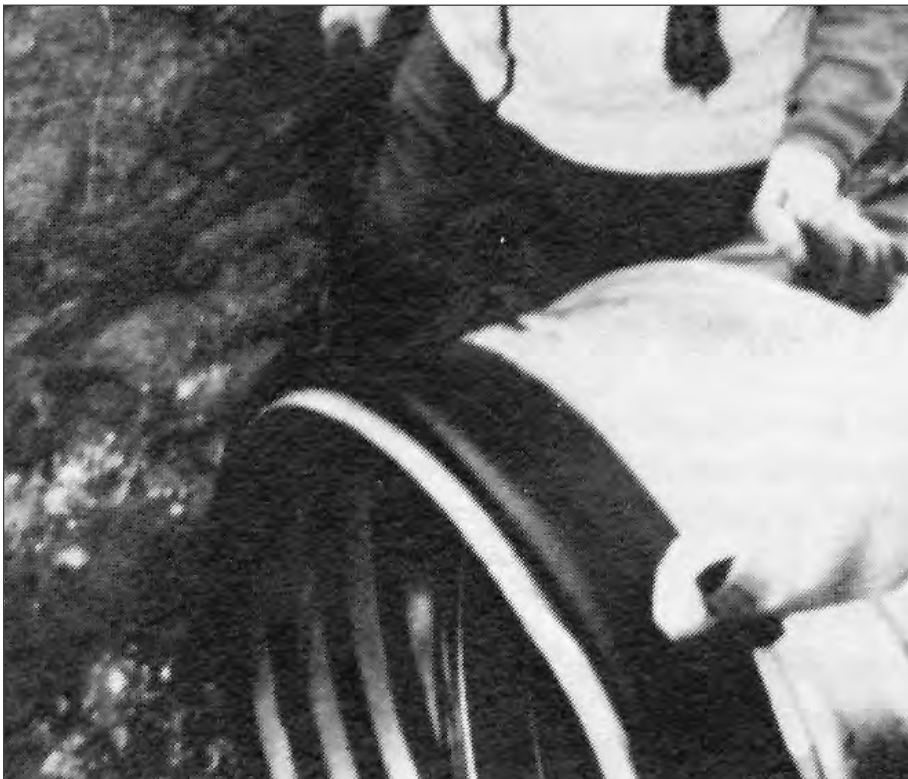
■ A flat gasket rolled back over itself ready to receive the next section of pipe.
