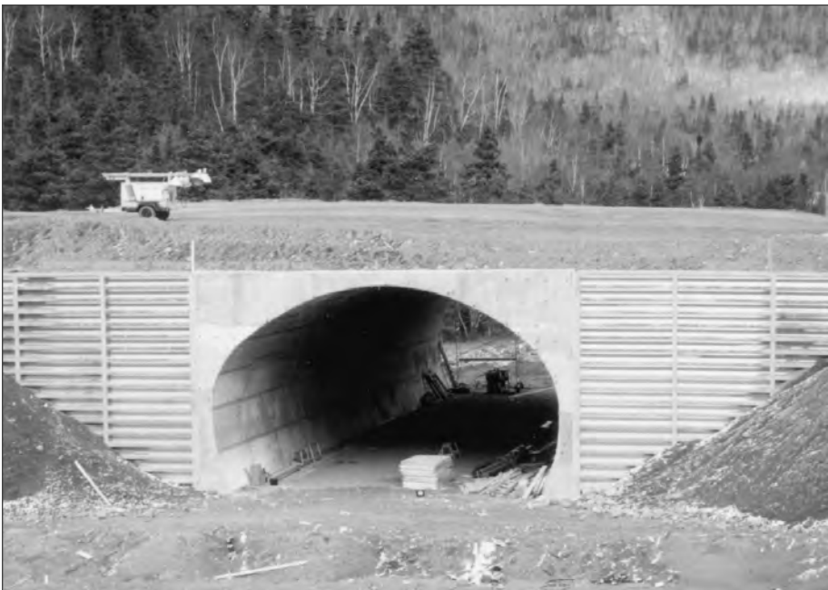
■ Long span high profile arch with concrete and bin-type retaining wall headwall.
