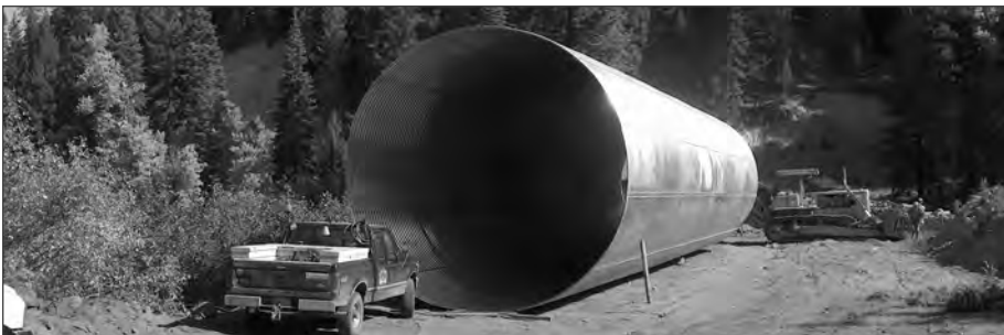
■ Fish Passage Project on the Mc Cloud River under the Mc Cloud Rail Road in Northern California. 16 foot and 20 foot diameter structural plate pipes.
