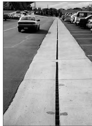
■ Slotted drain inlet pipe.
