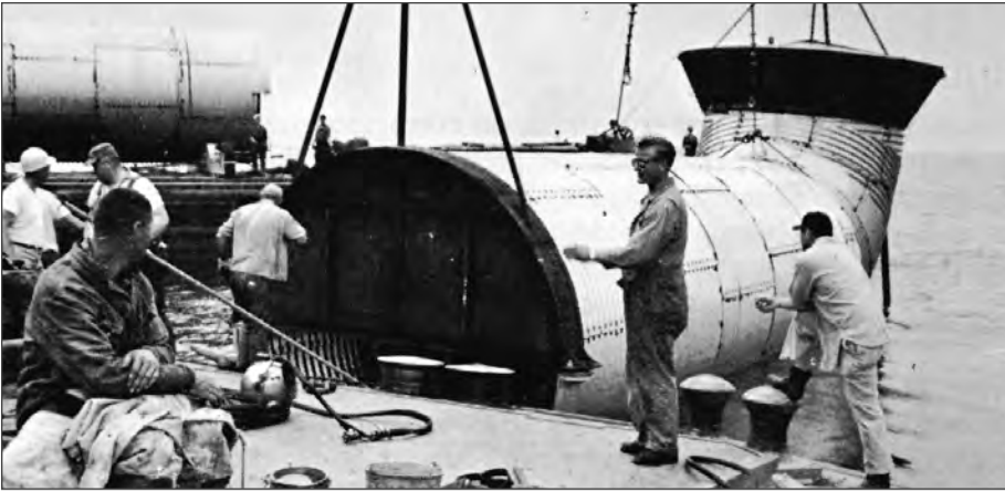
■ Special galvanized steel fitting for lake water intake of power station. Sealant ribbons were used on all seams. Divers made under water bolted connection between sections.
