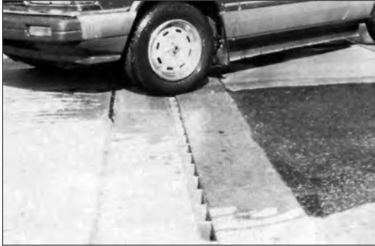
■ Slotted drain inlet pipe.
