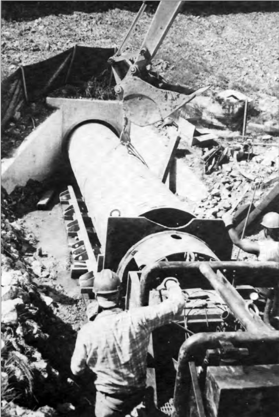
■ Figure 11.1 48 inch diameter CSP being used to slip line failed 54 inch diameter concrete pipe. Class 5, on partially constructed PA DOT Project – Southern Expressway – near the Pittsburgh Airport.
