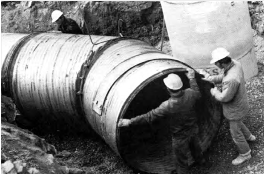
■ Figure 10.14 Pre-fabricated miter section of CSP is lowered into place to match bend in trench.
